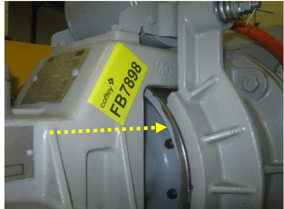
Photograph 2. Level 4: Lift Motor room; Lift Motor L.M 17 ('Elemol') - Brake callipers with compound brake shoes (Refer to sample FB7898 - NAD).
