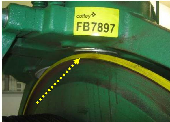
Photograph 1. Level 22: Lift Motor room; Lift Motor 4D ('M.X' 18 Lift Hoist') - Piston operated hydraulic brakes with compound brake linings (Refer to sample FB7897 - NAD).
